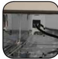
Interior Electrical Outlet
