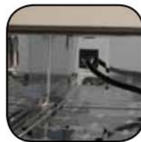
Interior Electrical Outlet
